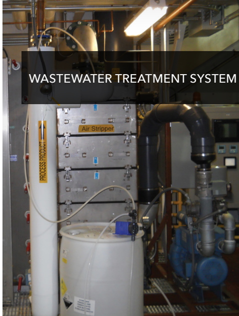
PFAS SOURCE TREATMENT SYSTEM
